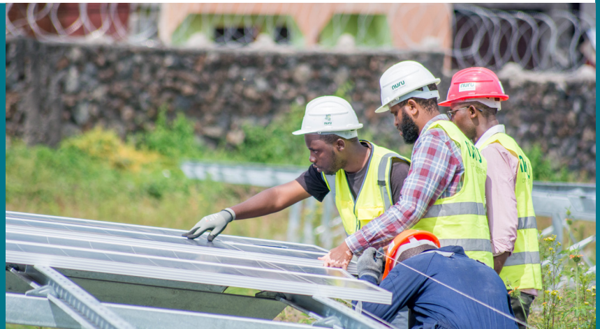
Above: Nuru's 1.3MW mini-grid deployment in Goma
